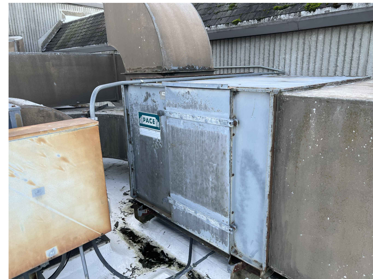
3 MD1.3 EXISTING AUX GYM RETURN AIR UNIT (RF-1)
