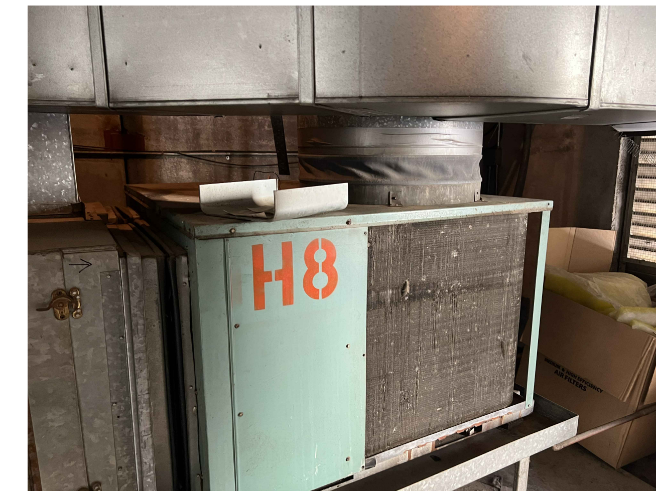
4 EXISTING CHORAL ROOM HEAT PUMP (HP-1)
