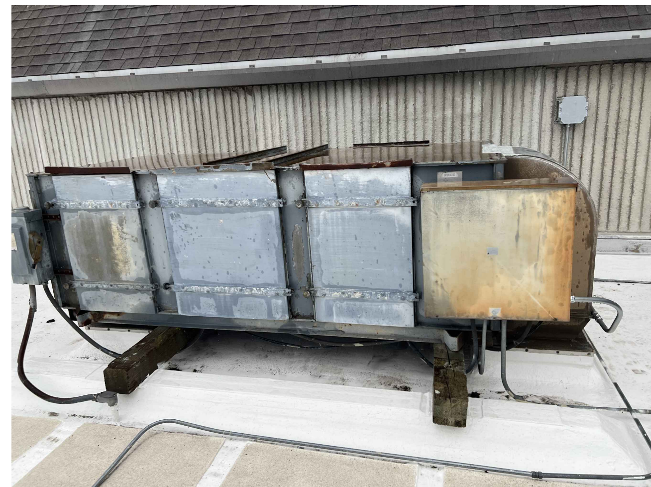
1 MD1.3 EXISTING GIRLS LOCKER ROOM UNIT (AHU-4)
