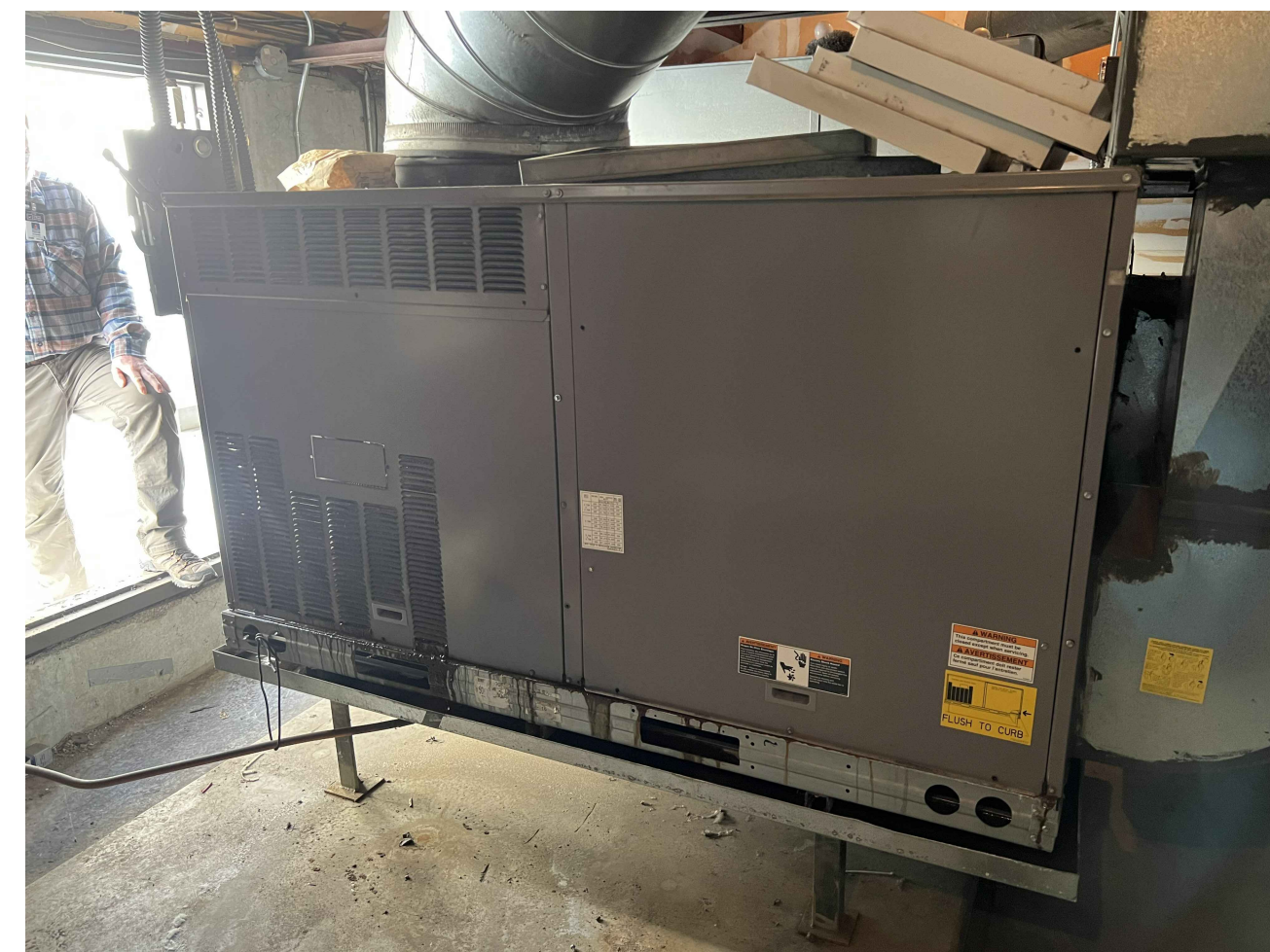
2 EXISTING BAND ROOM HEAT PUMP (HP-2)
