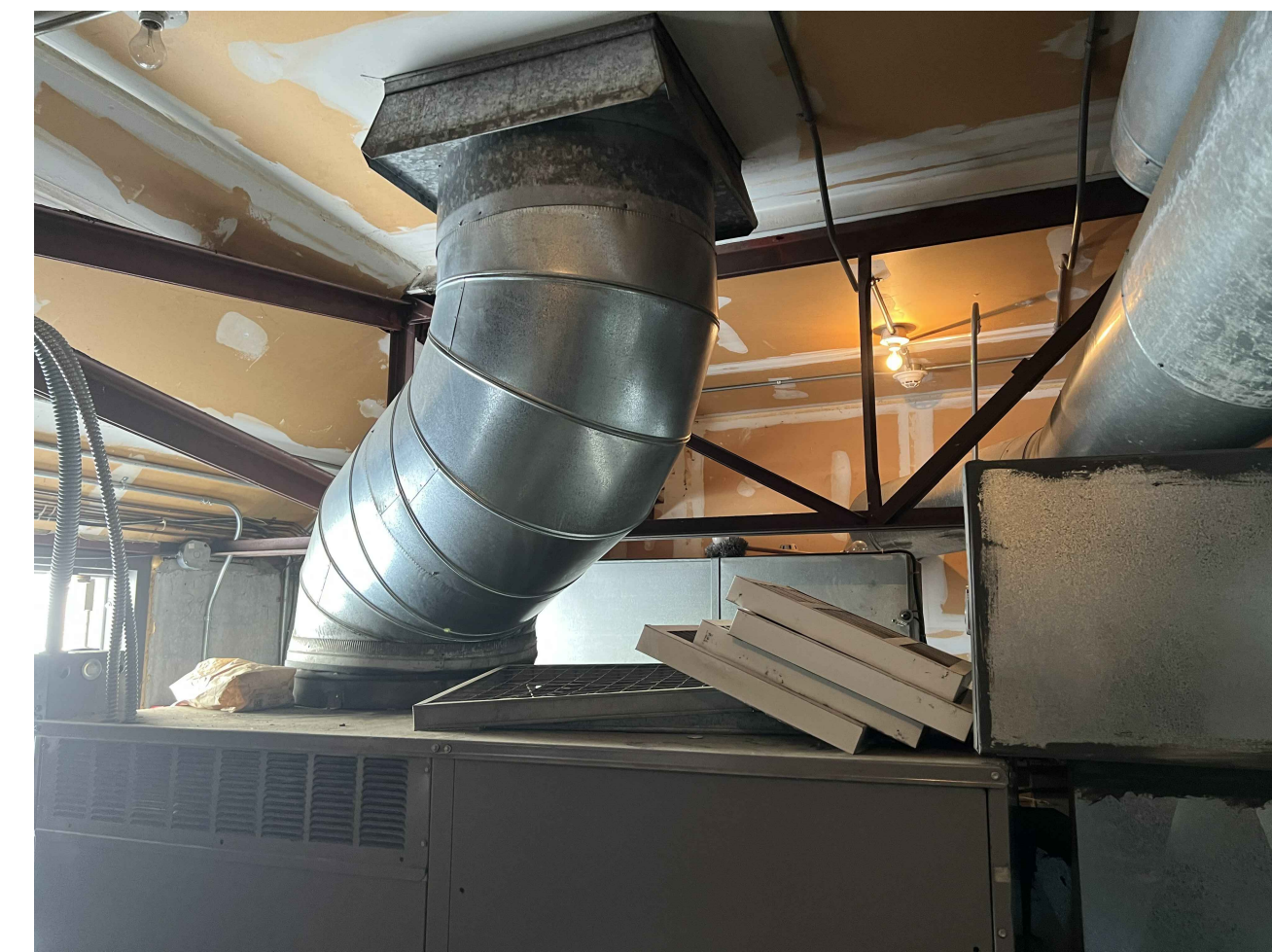
3 EXISTING HP-2 CONDENSER DUCT DISCHARGE
