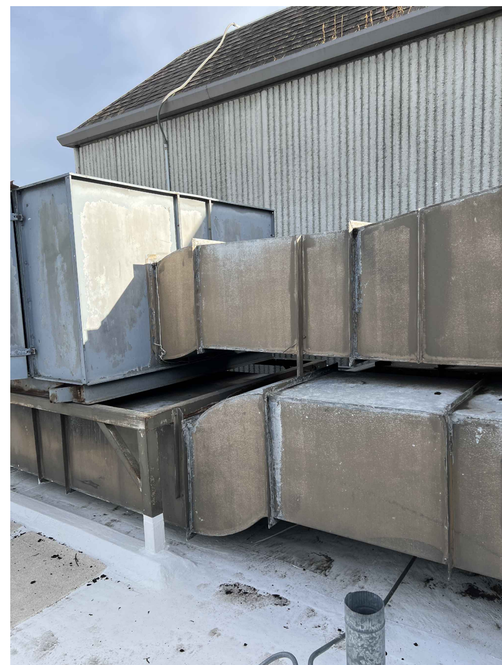
6 MD1.3 EXISTING DUCTWORK - GYM (NORTH) AIR HANDLING UNIT (AHU-1A)
