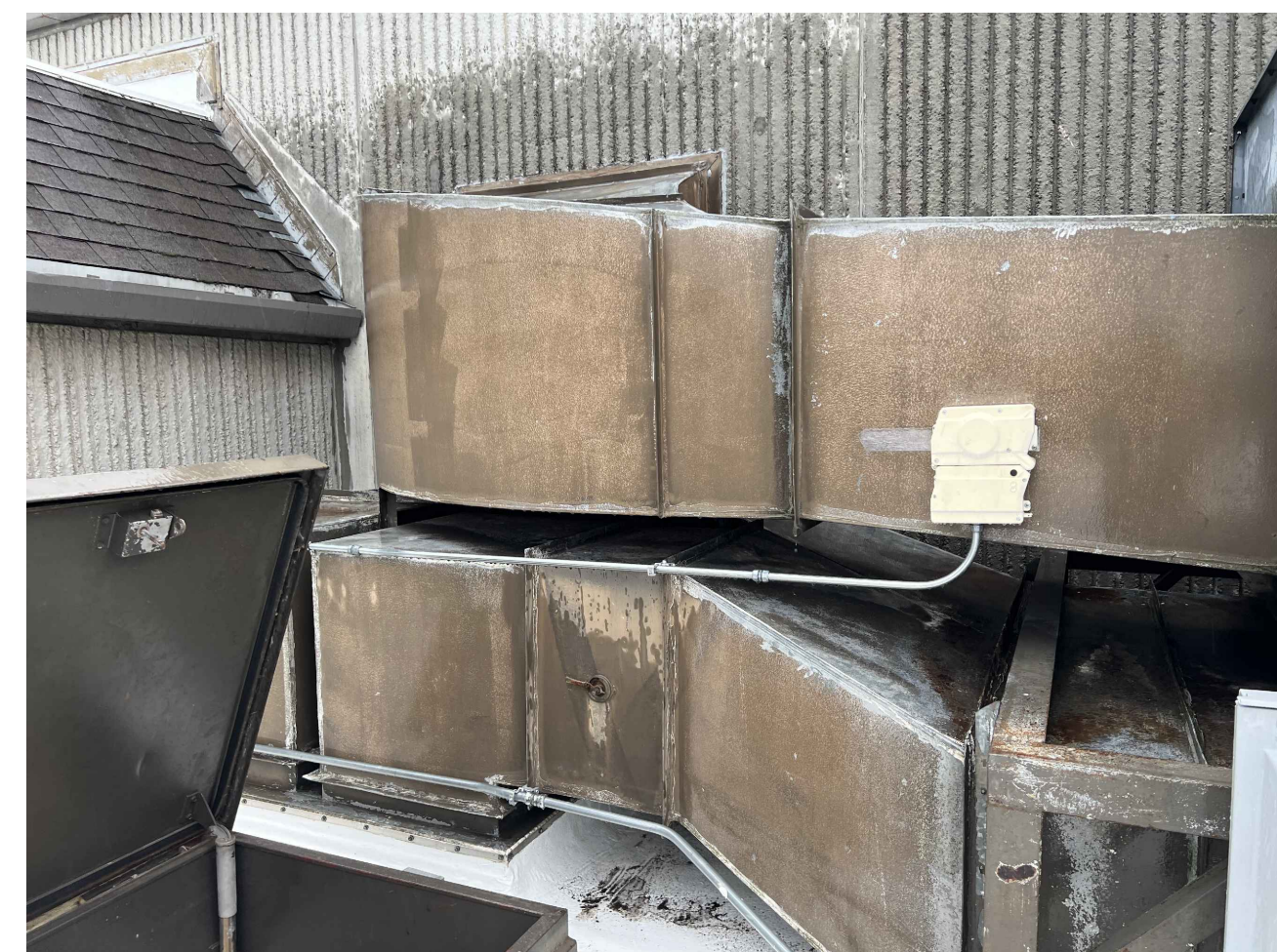
5 MD1.3 EXISTING DUCTWORK - GYM (SOUTH) AIR HANDLING UNIT (AHU-1B)
