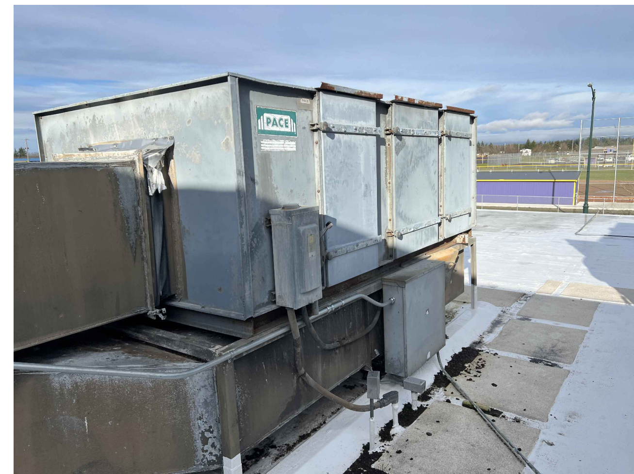
4 MD1.3 EXISTING AUX GYM AIR HANDLING UNIT (AHU-2)
